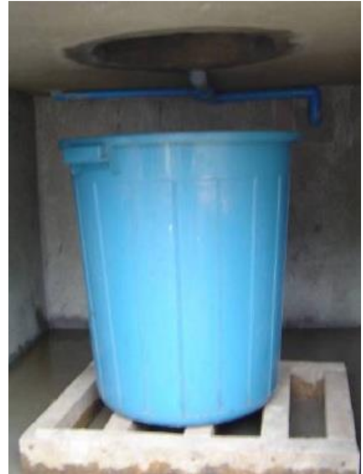
Drums for collection and storage of faeces, Philippines
