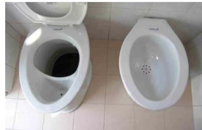
Drums for collection and storage of faeces and interior view of Single-Vault UDDTs
