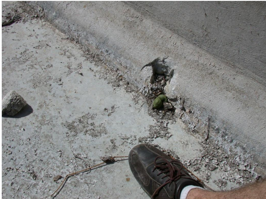
Figure 2: Spalling at the wall-floor interface in an unfinished constructed wetland
