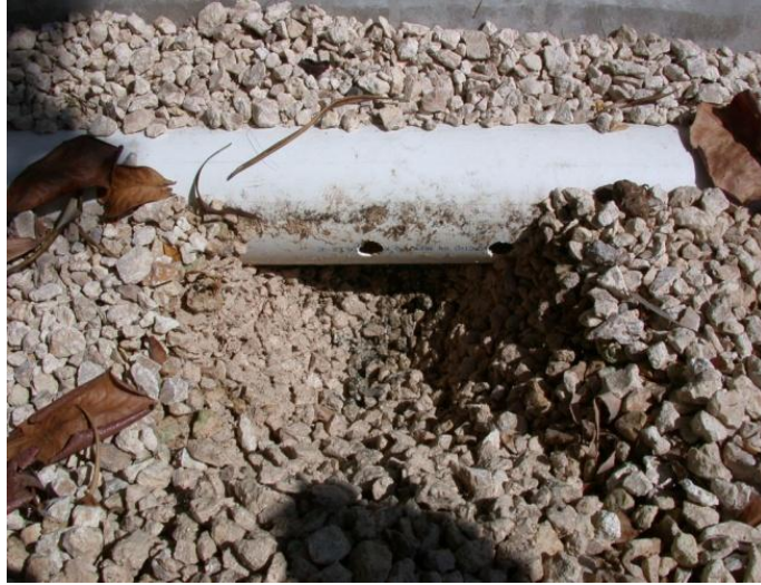
Figure 5: Larger aggregate at Villas Flamingo wetland. Spreader pipe exposed to show holes meant for dispersal of wastewater.
