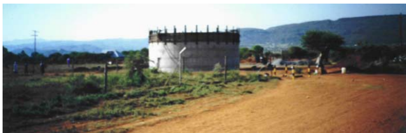
Figure 21: water reservoir under construction for a water supply project in Mohlaletse village
