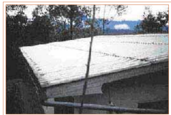
A typical corrugated iron steel roof showing guttering Ref: Intermediate Technology Development Group, UK
