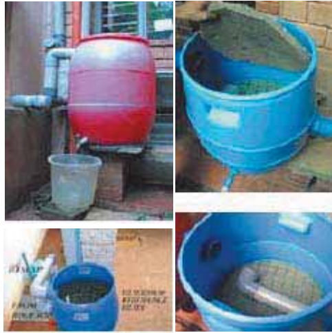
Drums - Filters and intermediate storage segregator
