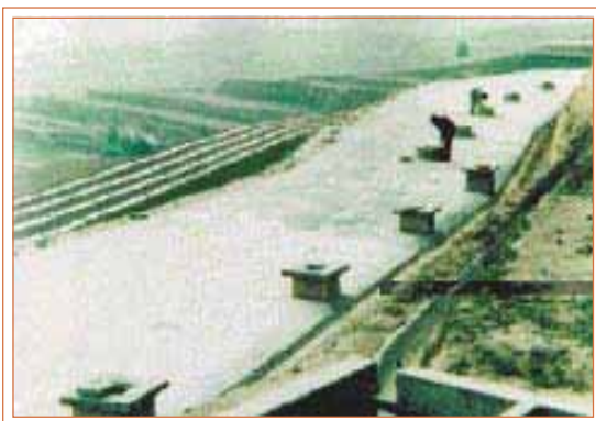
A group of water cellars and the rainwater collection field lined with concrete
