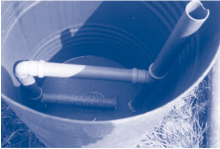
Pipe arrangement for sand filter
