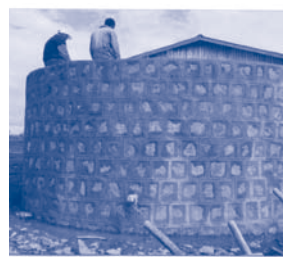
A communal masonry tank in Rural Ethiopia (Picture Water Action)
