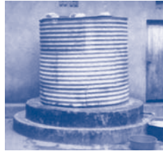
A corrugated steel tank in rural Uganda. Note the darker ring at the bottom of the tank – a concrete repair that is often needed (Picture: D. Rees)
