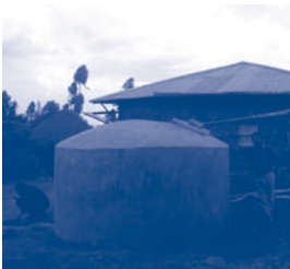
Household ferrocement tank in Ethiopia (Picture: S. Akhter)
