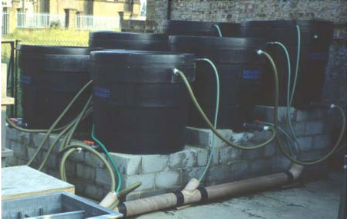
Plate 4.2: Filter tanks operating in series under gravity flow, at a pilot plant at Surbiton (London, UK).
