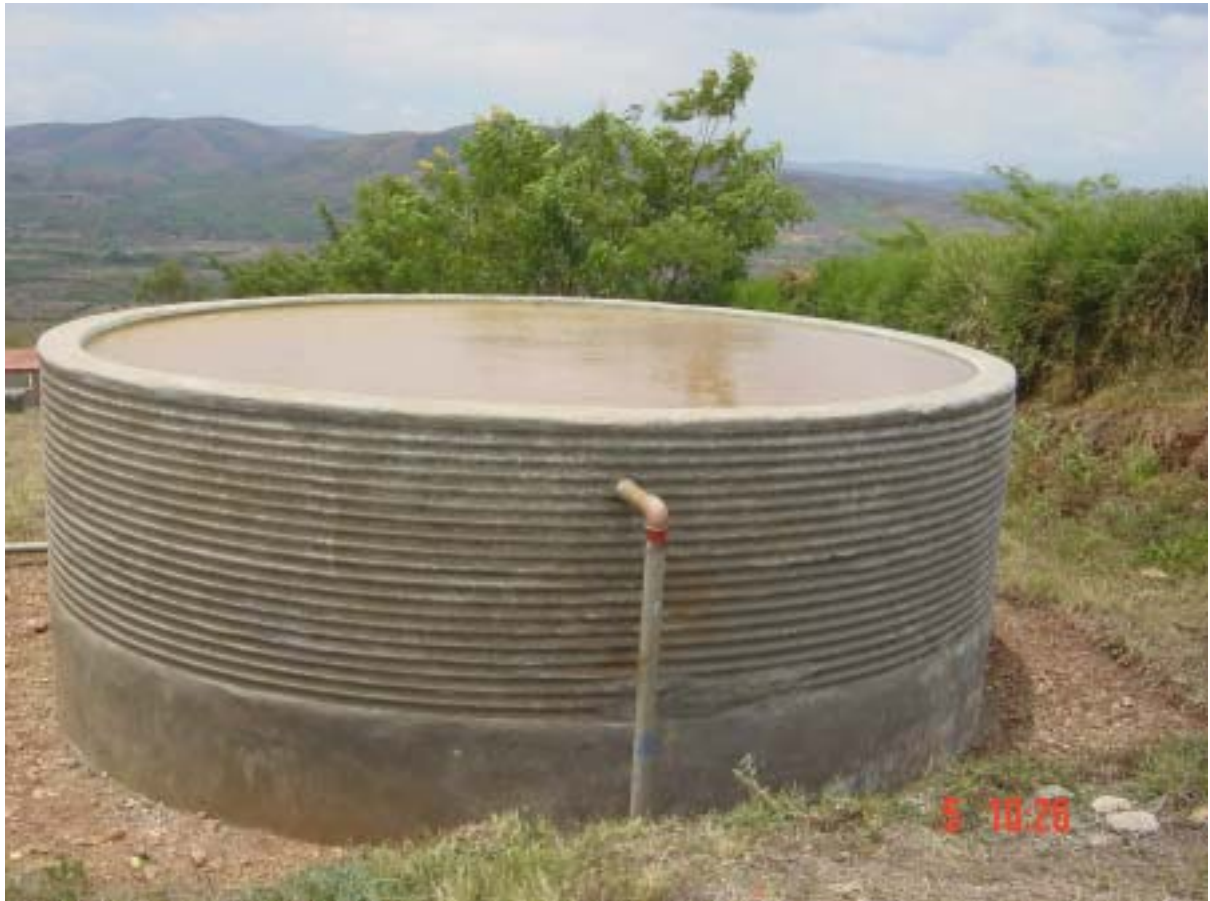
Plate Error! Style not defined..Error! Bookmark not defined.: Sedimentation Tank (50m 3 ) at the Nyabwishongwezi Water Treatment Plant, Umatara, Rwanda
