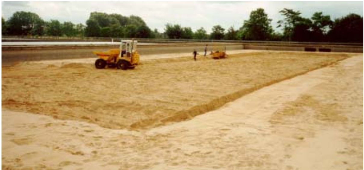
Plate 5.4: Re-sanding a SSF at the Ashford Common Advanced Water Treatment Works in London (UK).
