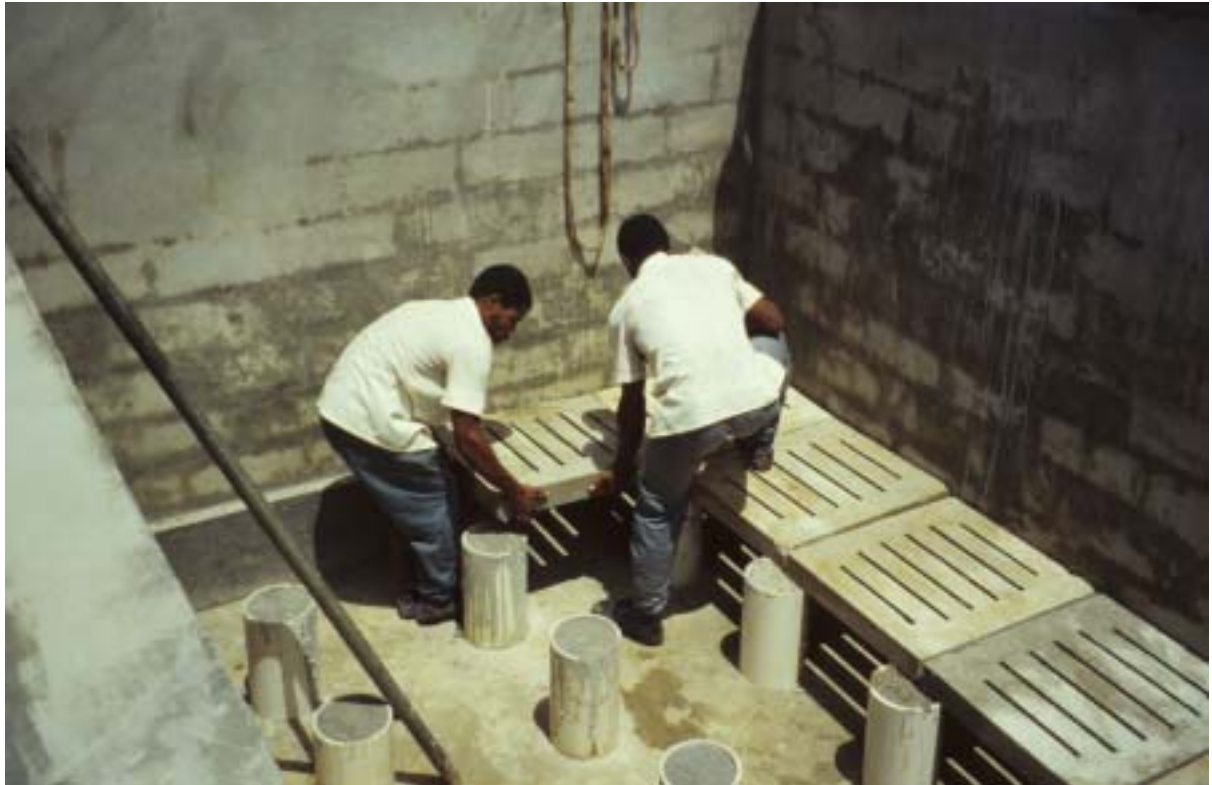
Plate 4.10: Laying under-drainage for a pre-filter at the Dennery Water Treatment Plant in St Lucia (also suitable for SSF under-drainage)
