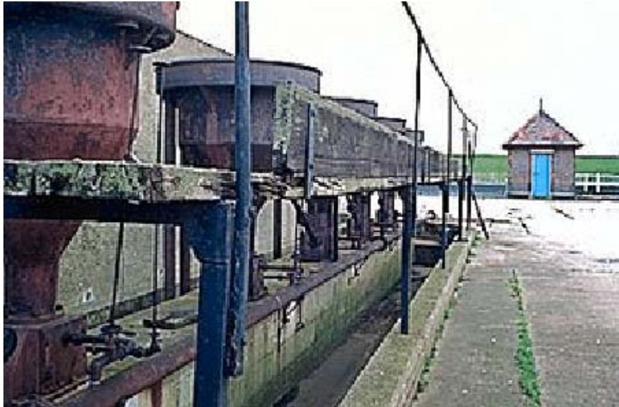
Plate 5.6: Bottle washers used to wash sand at a London SSF works
