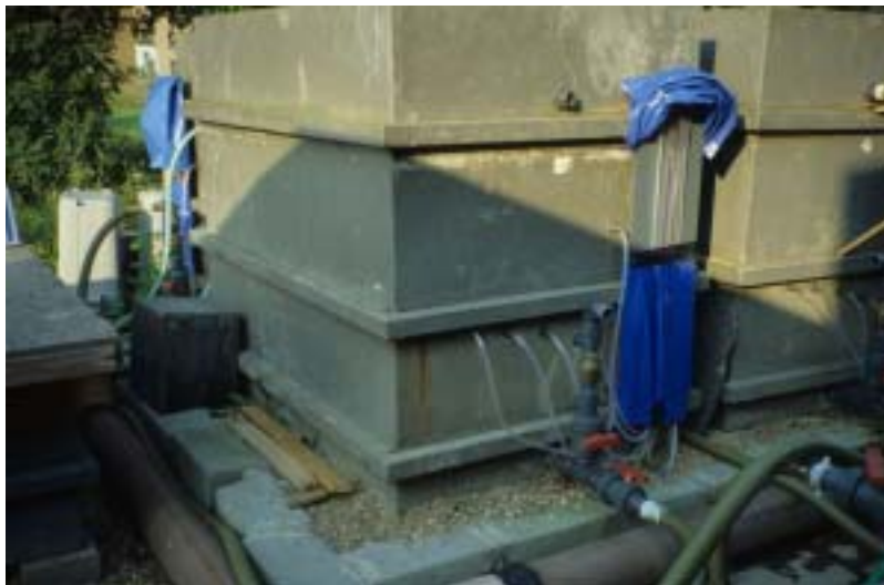
Plate Error! Style not defined..Error! Bookmark not defined.: Manometer tubes exiting a filter at Surbiton (London, UK). Note their arrangement to enable headloss measurement and also their protection against sunlight exposure.
