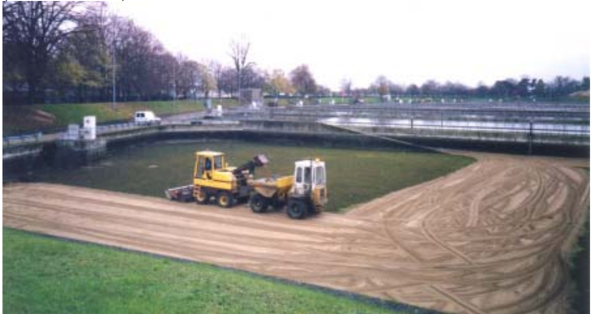
Plate 5.2: Mechanically skimming a SSF at the Hampton Advanced Water Treatment Works in London (UK).
