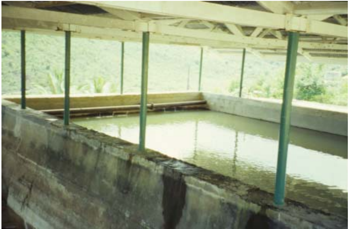
Plate 4.15: Shaded SSF for a community scale SSF at the Dennery Water Treatment Plant, St Lucia
