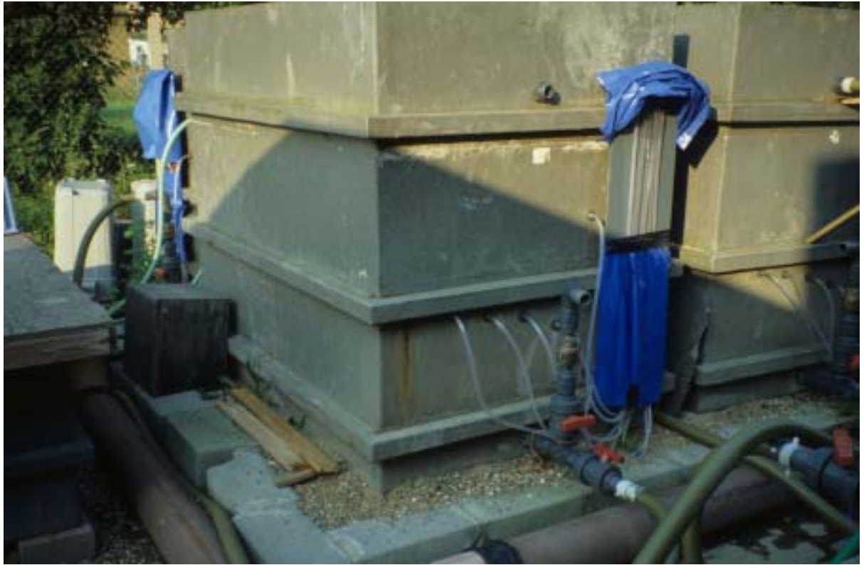
Plate 3.4: Manometer tubes exiting a filter at Surbiton (London, UK). Note their arrangement to enable headloss measurement and also their protection against sunlight exposure.
