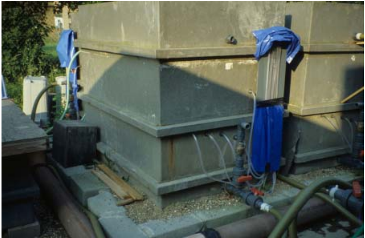
Plate 4.4: Manometer tubes exiting a filter at Surbiton (London, UK). Note their arrangement to enable headloss measurement and also their protection against sunlight exposure.
