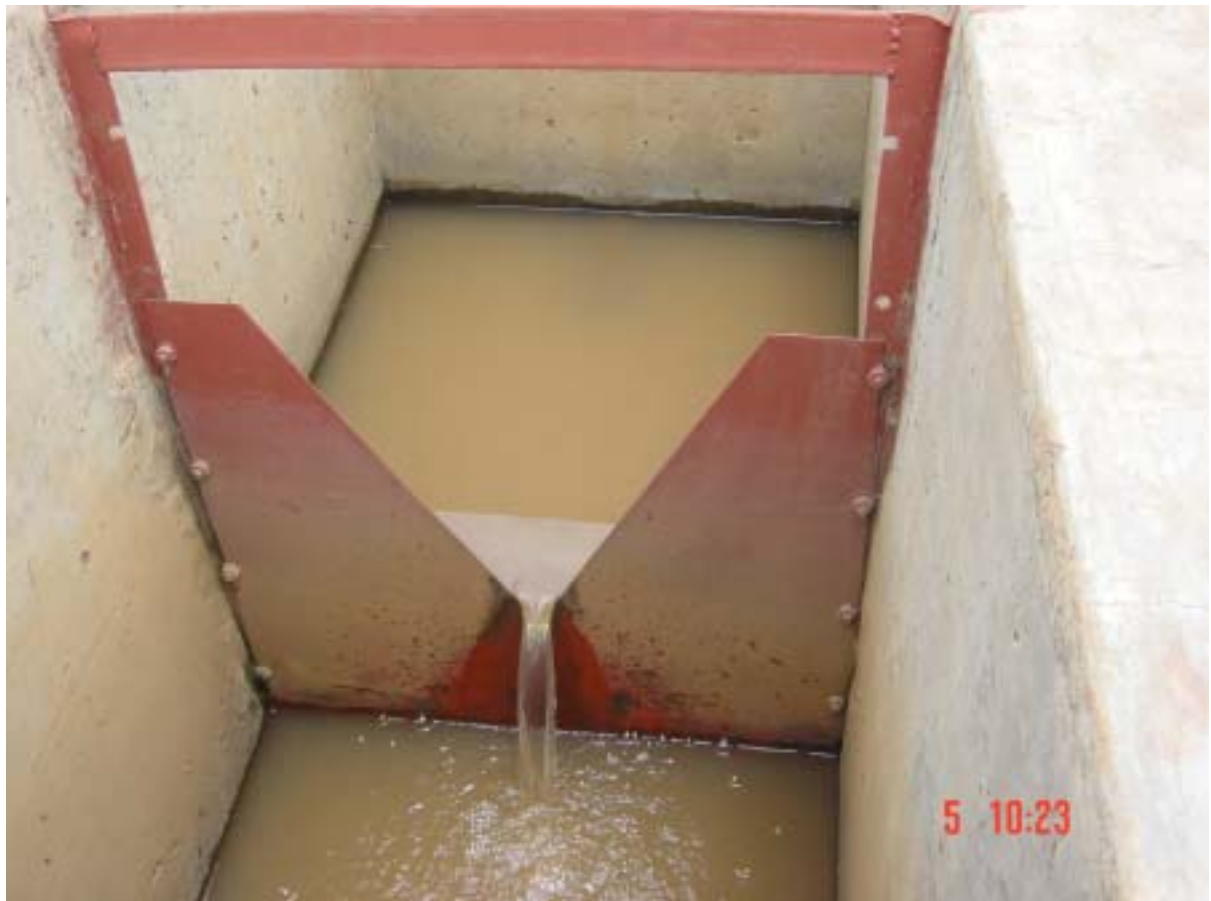
Plate 4.11: A 60° v-notch weir at the Nyabwishongwezi Water Treatment Plant, Umatara, Rwanda
