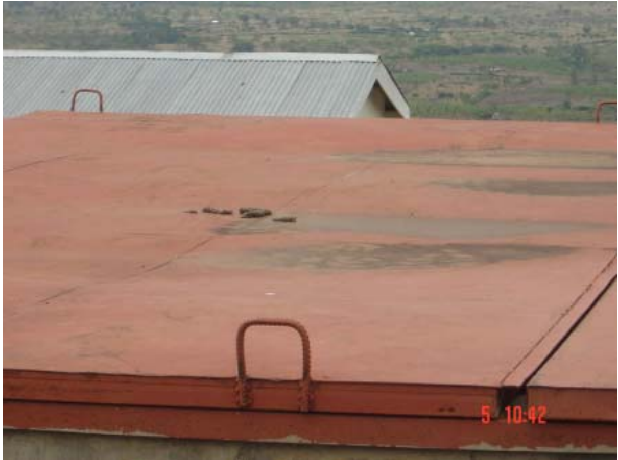
Plate 4.14: SSF covers at the Nyabwishongwezi Water Treatment Plant, Umatara, Rwanda
