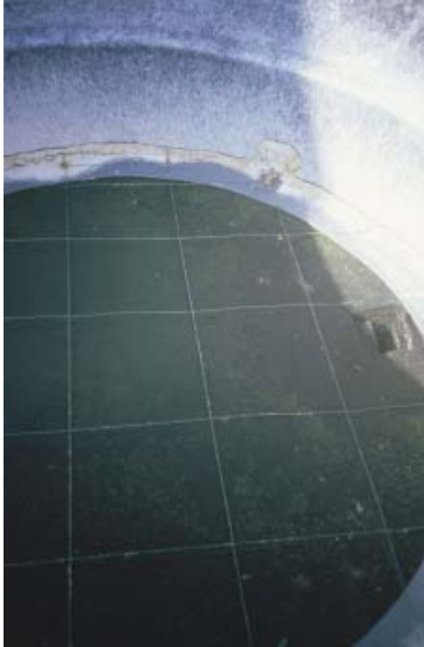
Plate 4.5: Surface Mat Installed onto a pilot scale SSF Bed at Shalford (Surrey, UK)
