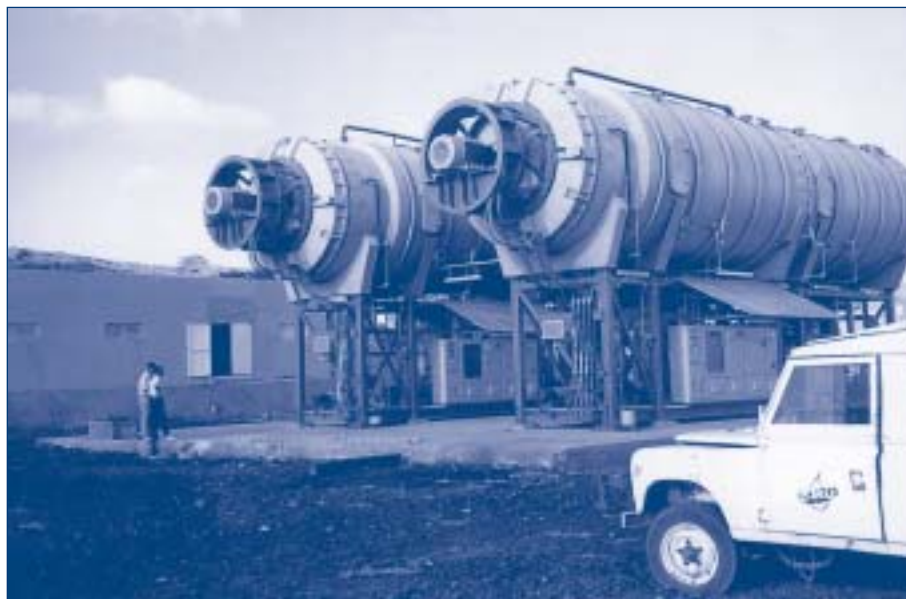
Fig. 18.6. Mechanical vapour compression (MVC) plant in Praia, Cape Verde (capacity: 2 \times 1250 \text{ m}^3/\text{day} ) (photograph by Jan C. Schippers)
