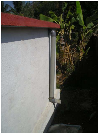
Fig 13: Overflow pipe with mesh
