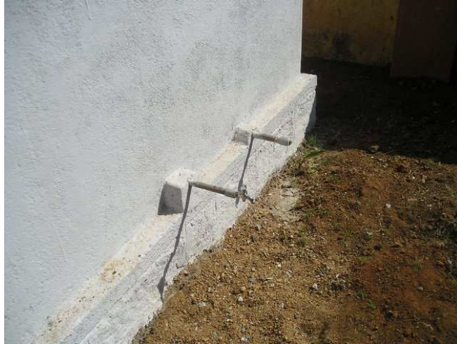
Fig 14: A tap and a drain out pipe firmly anchored to tank
