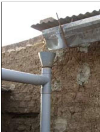
Rainwater delivery system, Burkina Faso (photo: RAIN Foundation).
