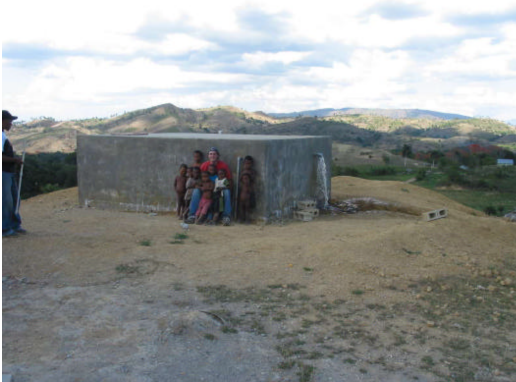
Figure 4.24 Water storage tank
