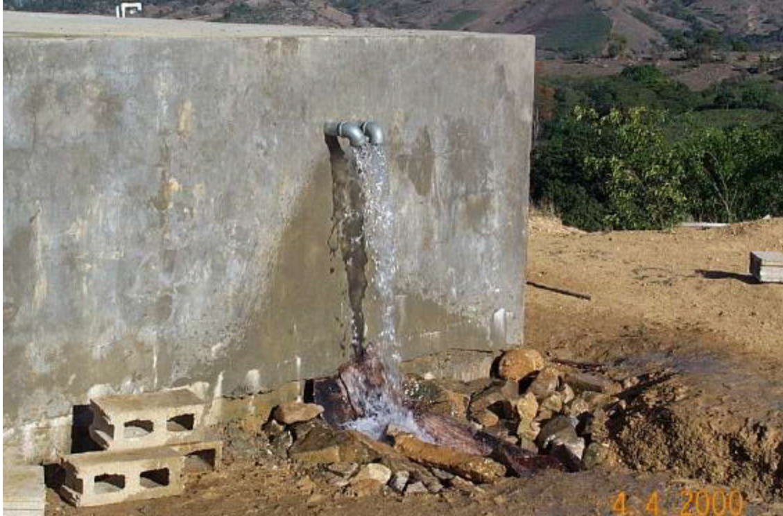
Figure 5.1 Water storage tank overflow – Unutilized volume above overflow.
