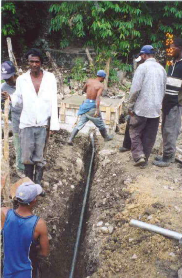
Figure 4.28 Transmission tank exit piping
