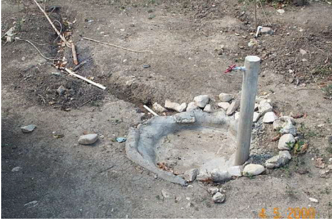
Figure 4.34 Installed tap stand
