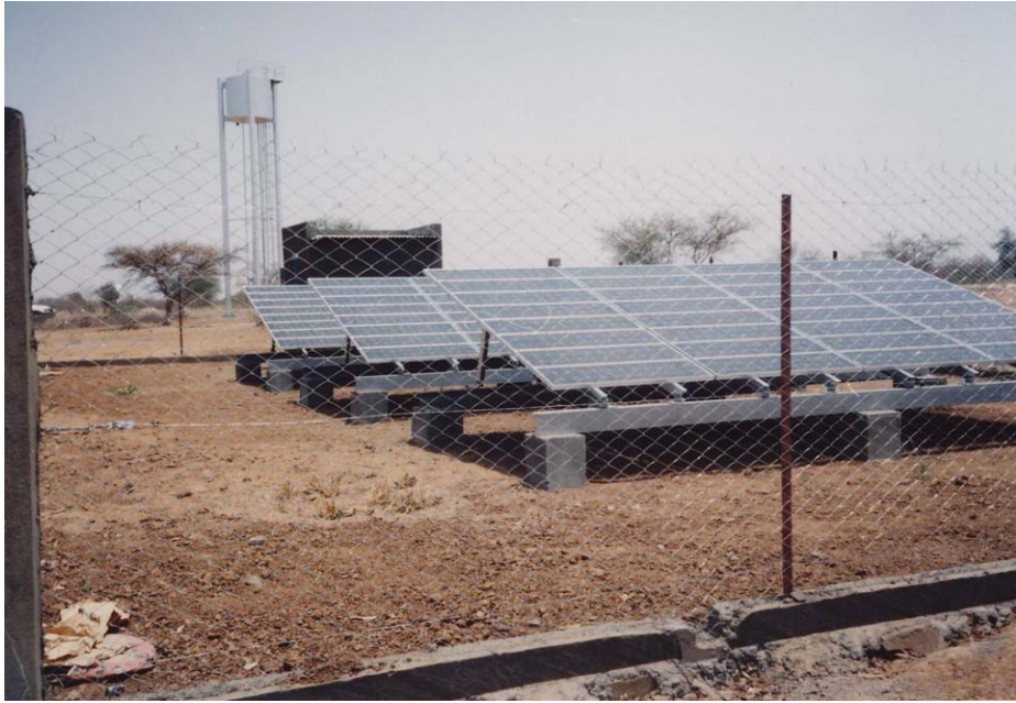
Photo 7.1: Solar power station for pumping
