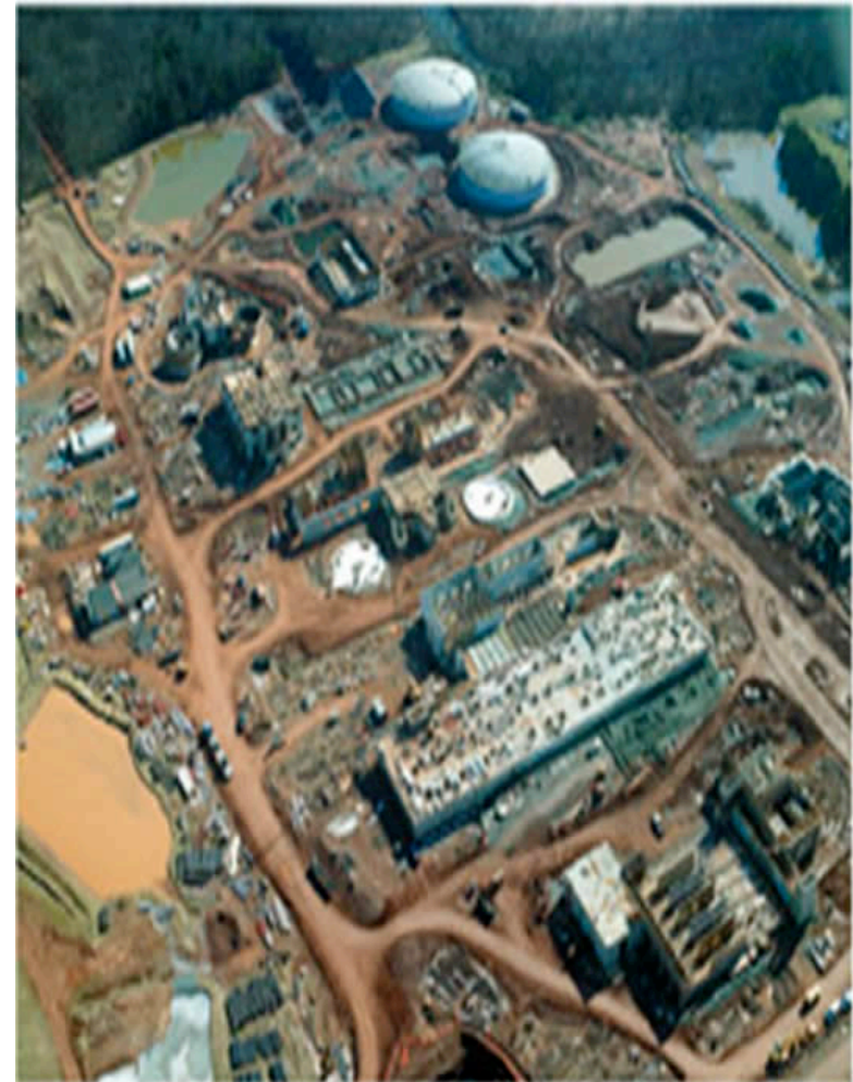
The Broad Run Water Reclamation Facility
