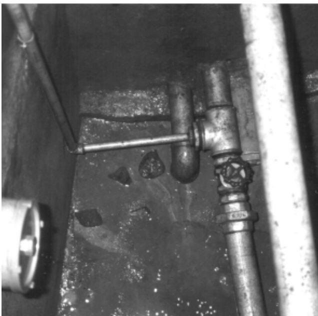
Easy accessible operation chamber – well maintained
