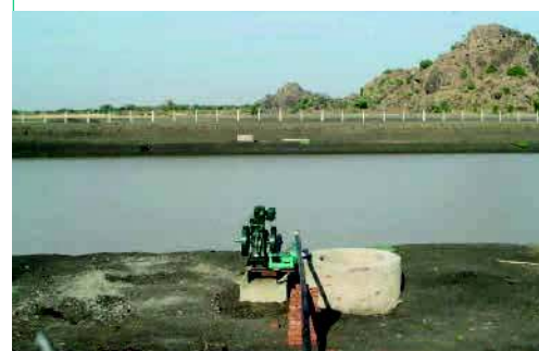
Excavated pond (improved hafir system) with water pump and sedimentation tank. (Ministries of Water Resources and Irrigation of Sudan and South Sudan, 2009)
