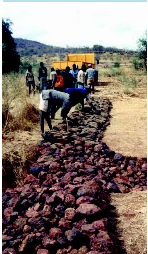
Constructing a permeable rock dam ( digue filtrante ) in Burkina Faso. (W. Critchley)
