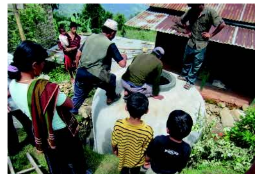
A rainwater storage tank constructed by householders in Nepal. (RAIN)
