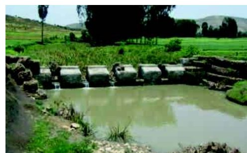
Check dam made of stone, concrete and gabion for irrigation purpose at the same time reducing the runoff velocity and enhancing gully rehabilitation. (E. Yazew)
