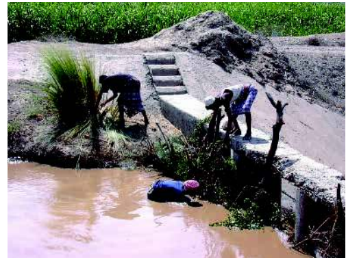
Blocking scour sluice on a modernised spate irrigation system in Yemen. (spate-irrigation.org)
