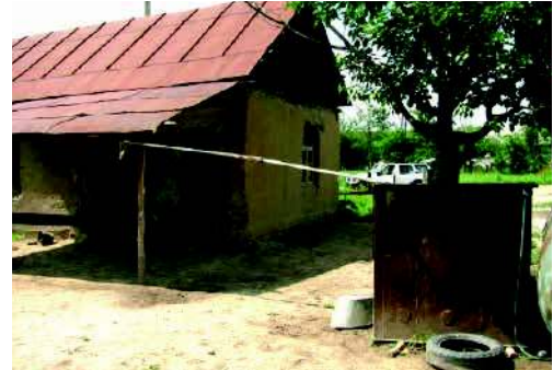
Example of RooftopWH in Kyrgyzstan. (L. Pluess, Helvetas)
