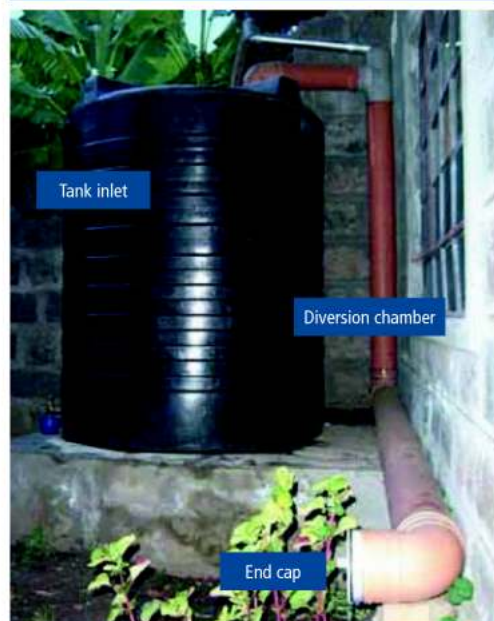
Plastic tank with a first flush system, Kenya (Stevenson, 2007 in Doyle, 2008).
