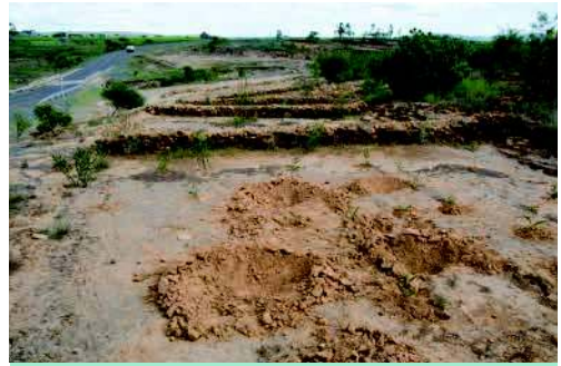
Road runoff harvesting system with macro- and microcatchments in Ethiopia. (HP. Liniger)
