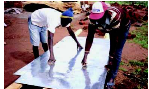
Manufacturing square-sectioned gutters from galvanized plain iron: shaping them with a piece of wood (Nissen-Petersen, 2007).
