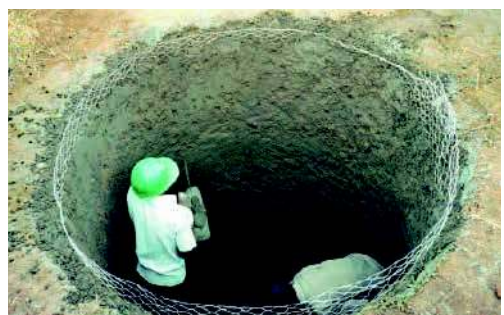
Underground tank for courtyard and road water harvesting, Kenya. This tank was equipped with a silt trap and used for storing runoff (Nissen-Petersen, 2007).
