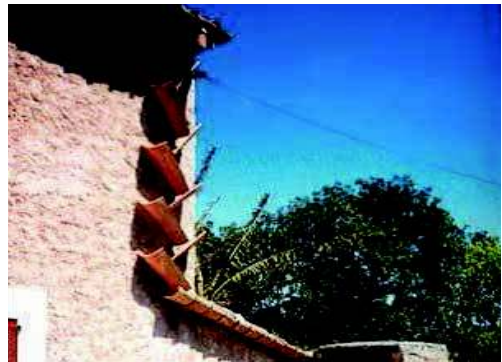
"Cascading gutters" of a RooftopWH system for domestic use in Mallorca, Spain (Barron, 2009).
