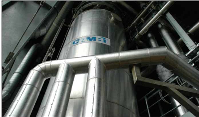
One of the two THP reactors. Photo by Cambi AS
