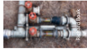
Picture 5: Flow meter
