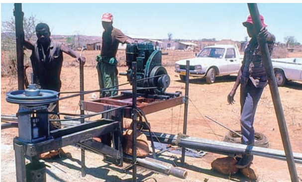
Figure 17: A test-pumping rig in operation (it consists of a belt-driven mechanical rotary (Mono) pump), Zimbabwe
