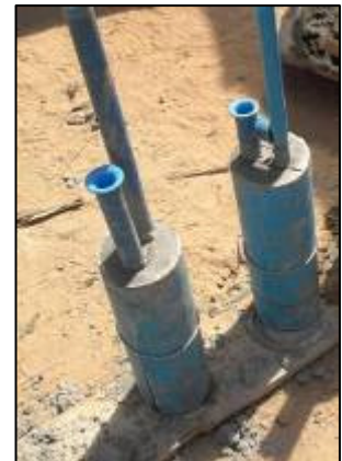
Concrete guide boxes
