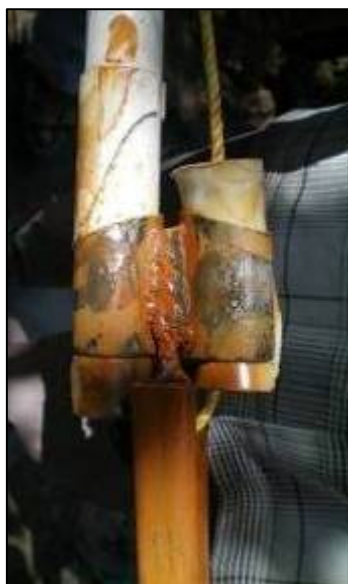
Corrosion on a guide box
