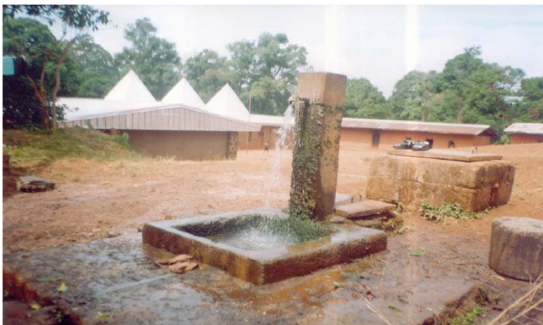
Picture of poorly managed standpipe.
