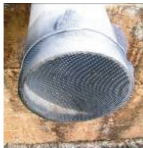
Tank overflow covered with fine mesh
