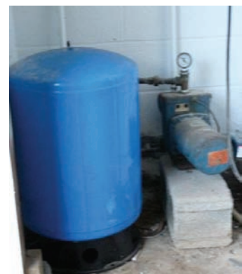
Figure 26 Pressure tank (left) and pump
