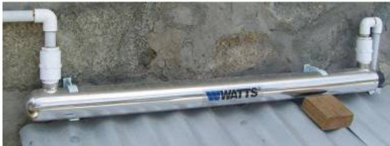
Figure 32 A typical ultra-violet lamp on a RWH installation (before entry to building)
