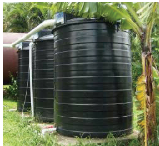
Figure 18 Multiple PVC tanks for rainwater storage
