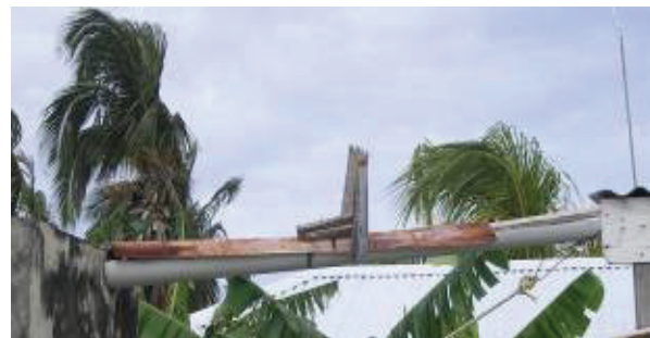
Figure 30 An example of a rat guard along a gutter to a storage tank in the Grenadines
