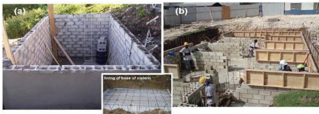
Figure 21 Typical block-type cisterns under construction (a) household (b) commercial applications (photos courtesy Dr. Everson Peters and Andrew Hutchinson)
