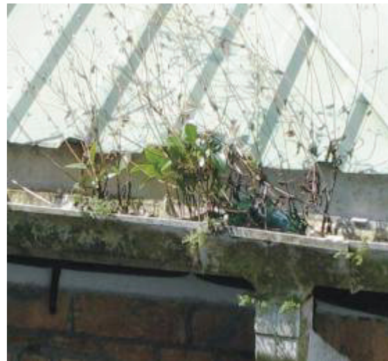
Figure 31 An example of a poorly-maintained gutter
