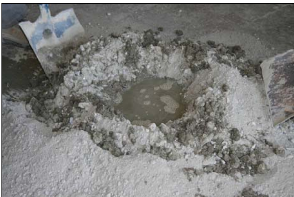
Mix the dry ingredients together using a shovel. Make a shallow hole in the centre and pour water into the hole. Mix thoroughly and continue to add water until it reaches the proper consistency.
