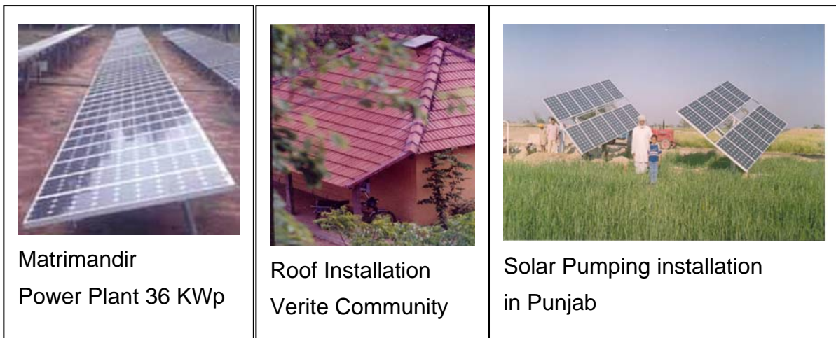
Different types of solar installations
