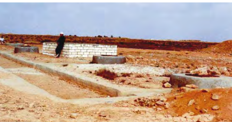
Newly built cistern in northwest Egypt, with approach channel and settling basin.
